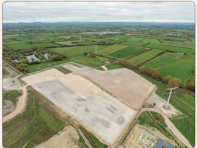
Groundwork underway for the National Grid Electricity Transmission (NGET) substation at the east of the site
